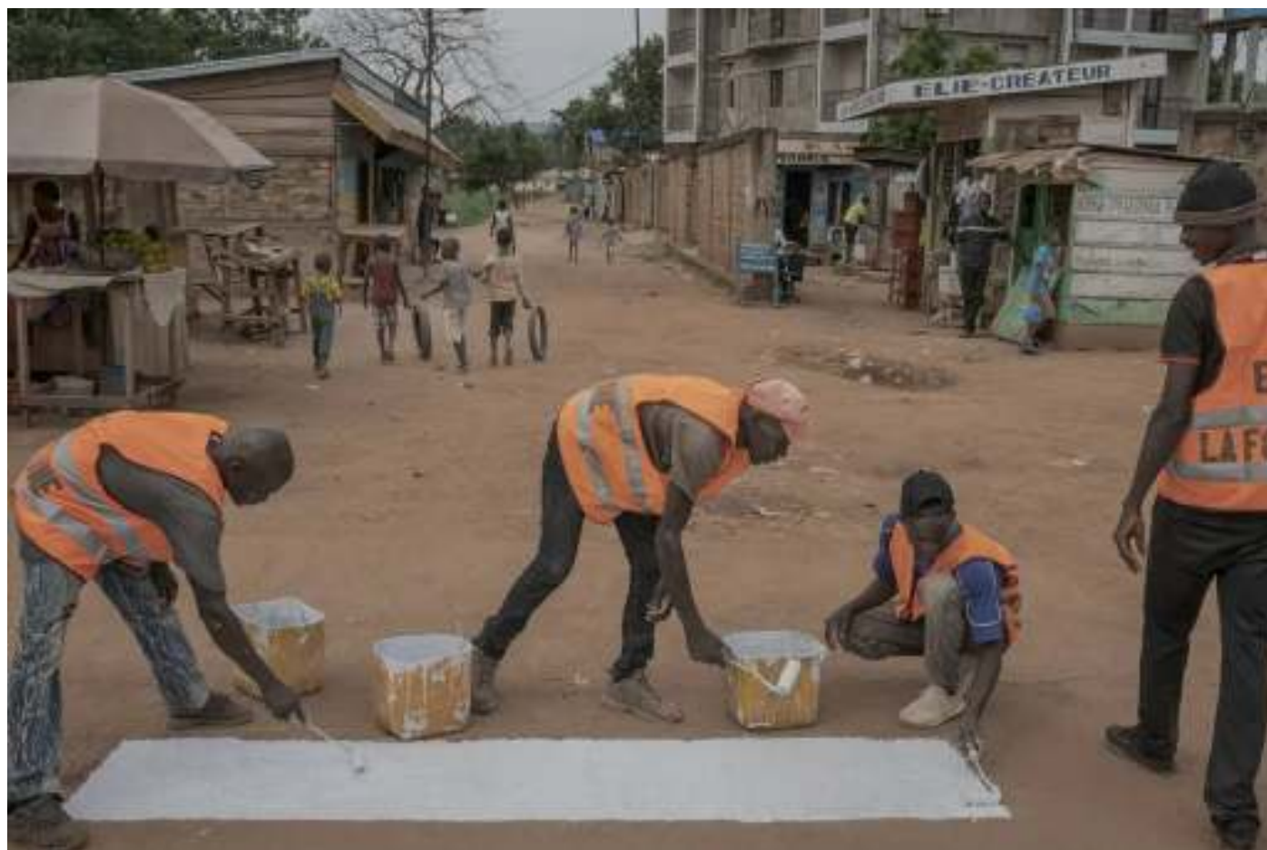
Workers painting a crosswalk in a residential neighborhood in October in Bangui.
